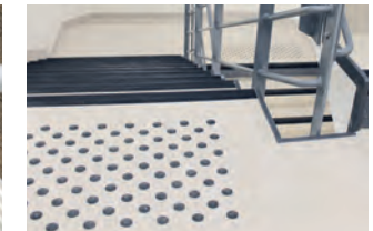
Tactile warning tiles for safety
