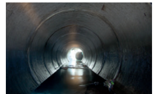
Sewage ducts and shafts
